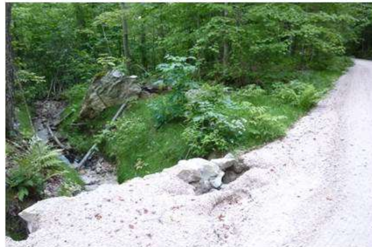
3. Erosion of road sediment from culvert header into tributary draining to Woodward Reservoir; site uphill from photo 1.
