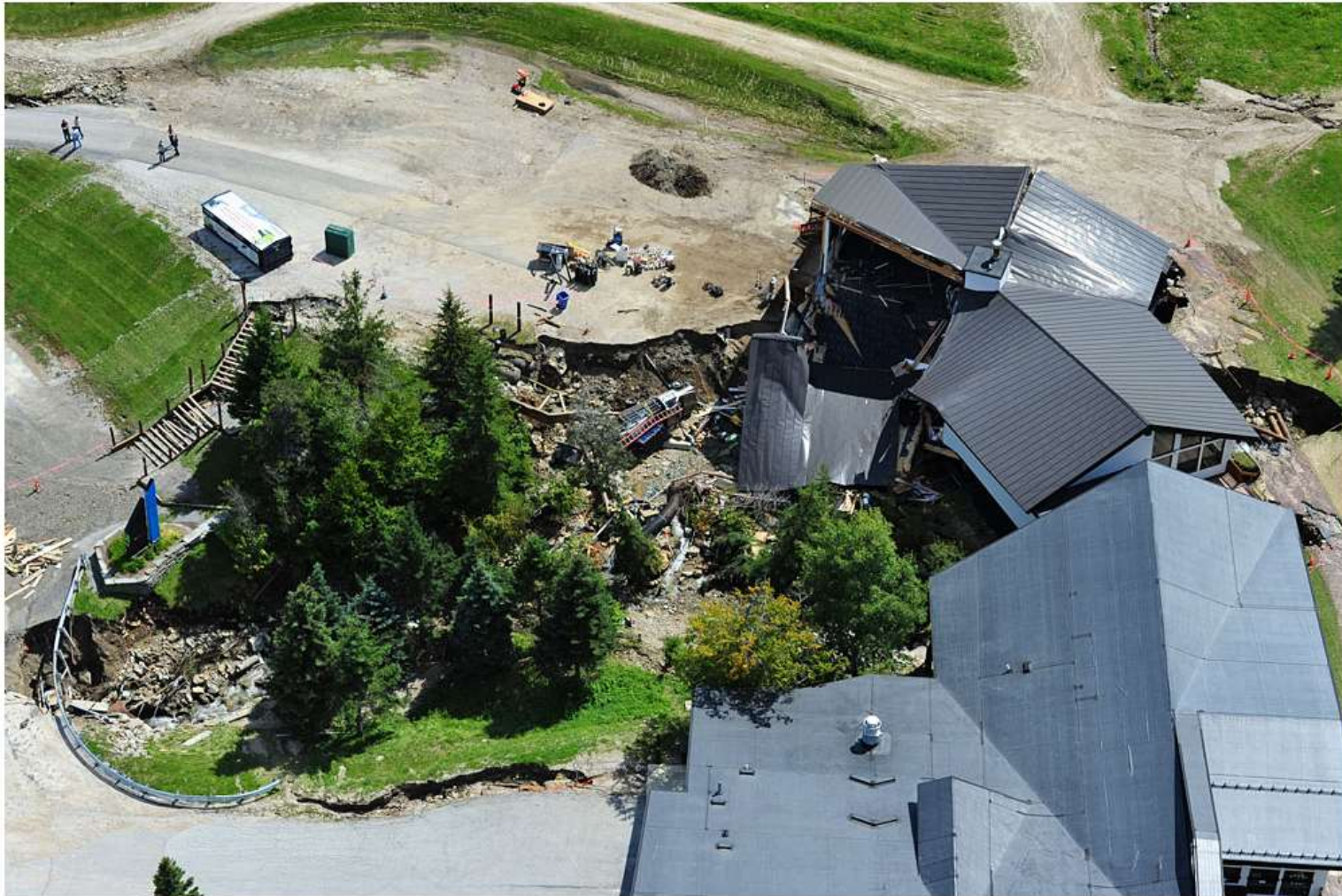
Photo 1. Partial collapse of K-1 base lodge, Superstar Pub addition, at Killington Resort – August 31, 2011. Building foundation and access road undermined by floodwaters from the Roaring Branch. Photo Credit: Lars Gange and Mansfield Heliflight
