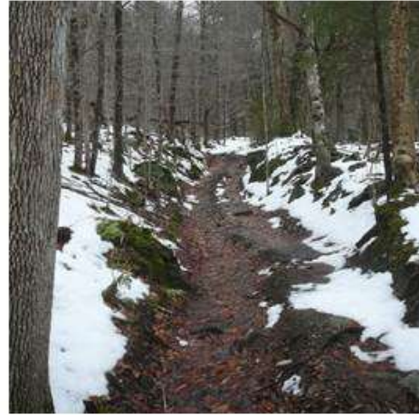
6. View uphill on narrow forest road that is channeling runoff; dugway banks are 5 ft high in sections.
