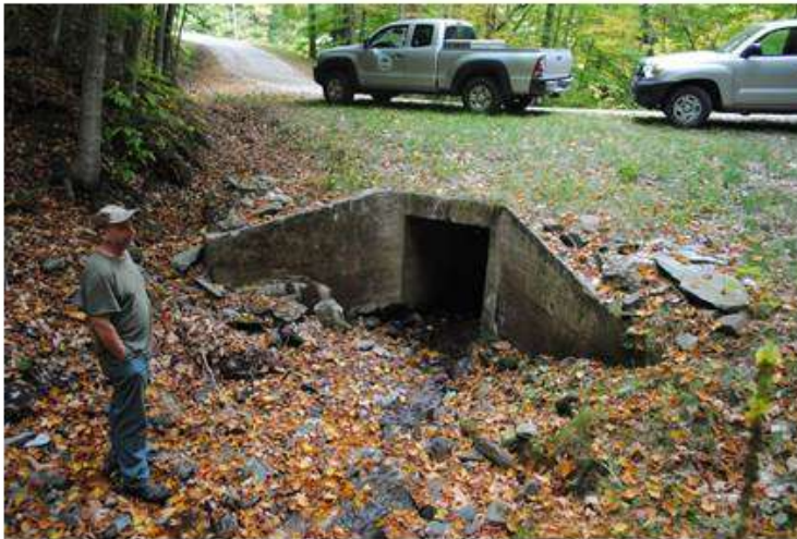
1. View downstream to box culvert crossing of Quarry Road over unnamed tributary to Pinney Hollow Brook.
