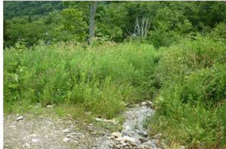
7. One of several water bars on maintenance road, draining to rock-lined detention areas, before discharging to Roaring Brook.
