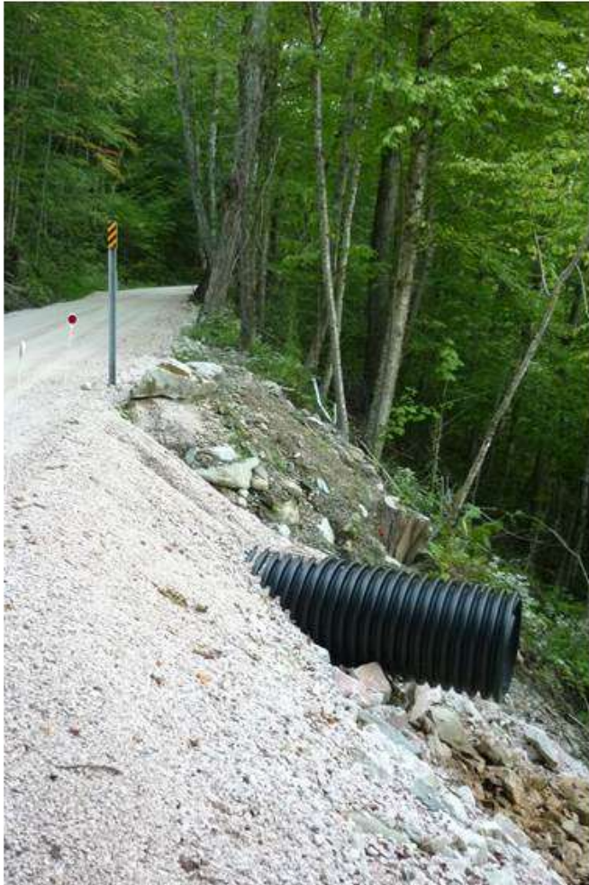
1. One-lane segment of CCC Road and stream crossing replaced after TS Irene on >25 % hillslopes through Northern Hardwood Seepage Forest.
