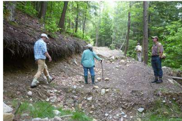
8. Forest road installed across >35% slopes, to access patch cuts. Steepness of hillsides and use of skidders necessitated wide road cuts. Steepness of road grade (>10%) required frequent water bars.
