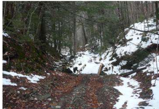
8. Road ditch directs runoff to the stream at the bridge crossing.
