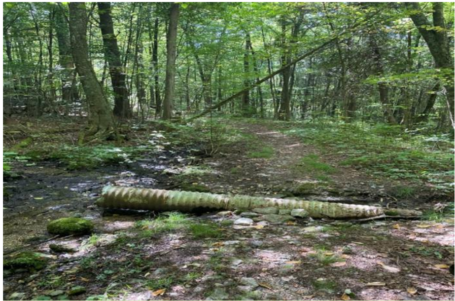
An old, non-functioning culvert along the mail trail at the Lands of the Watershed Center. This is one of 47 erosion control structures slated for improvement.
